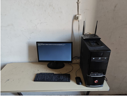
(a) Control room.
